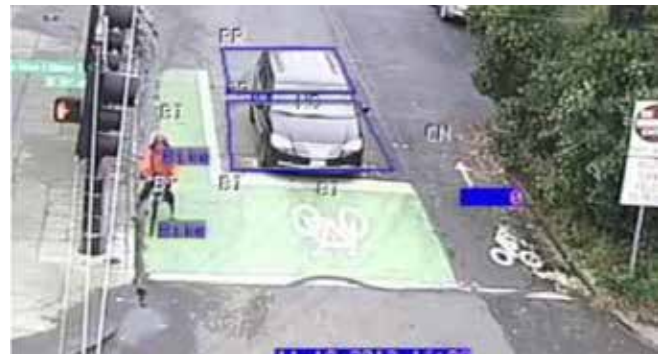
Traffic signal with video detection upgraded to detect and count bicyclists. SmartCycle software shown ( www.iteris.com )
